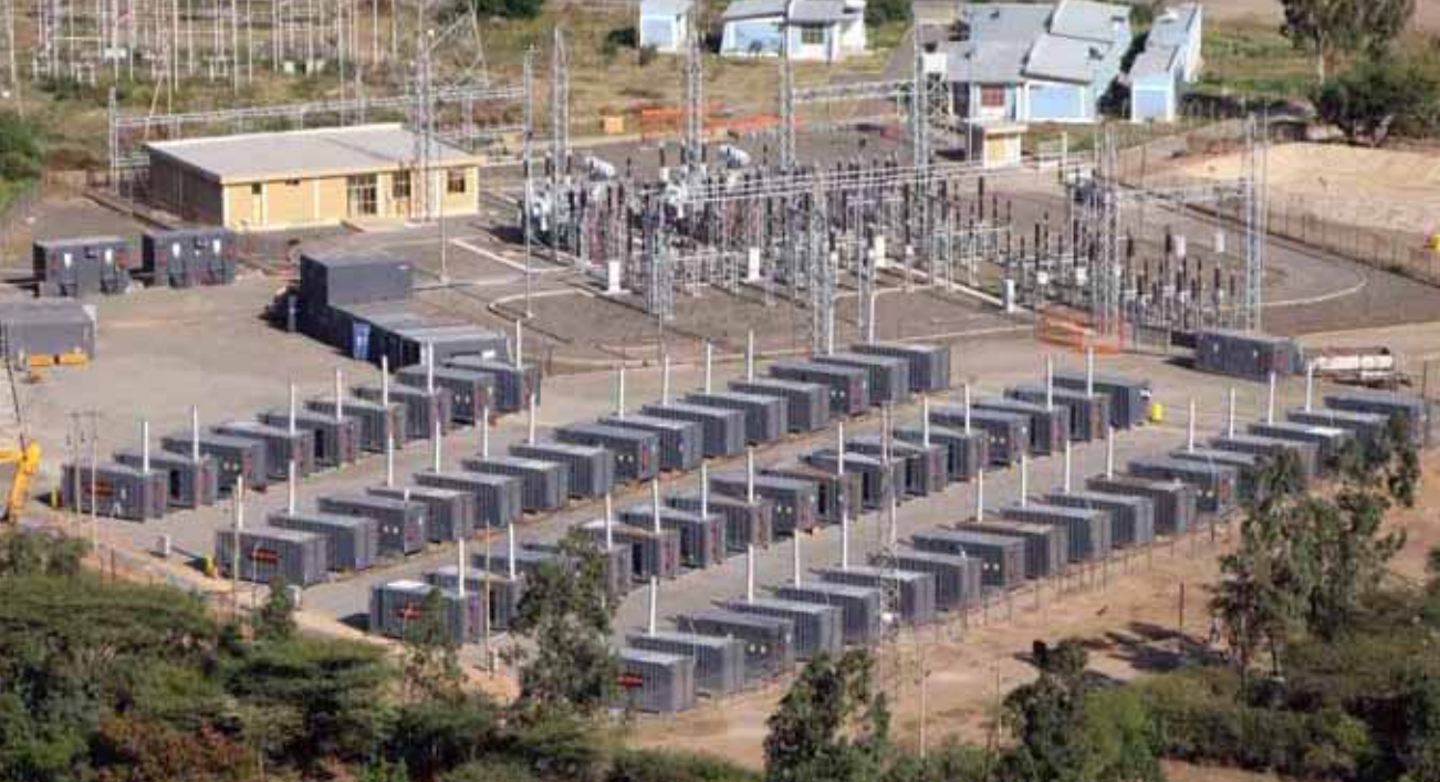
30 MW base load power to support the national grid, Ethiopia
